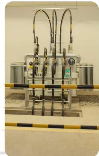
Electrical room Paseo San Francisco
