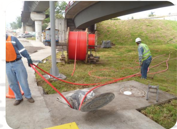
Underground transmission lines Bocatoma
